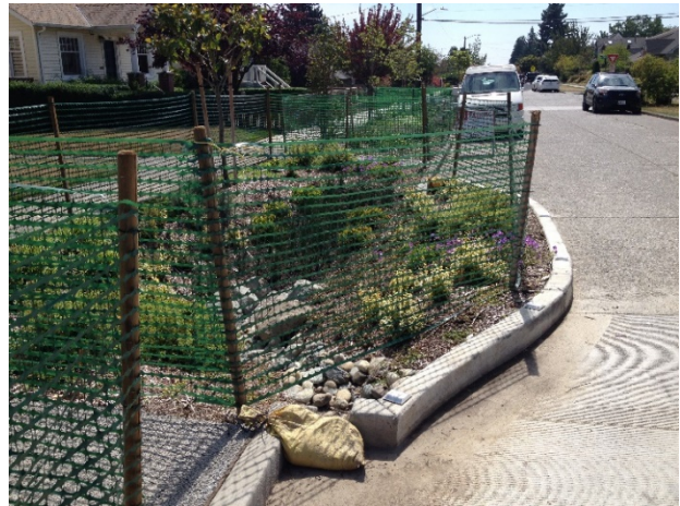
Sand bags prevent silt-laden flow from entering the bioretention facility. Green construction fencing prevents compaction due to foot traffic.
