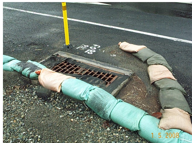
Temporary sand bags divert construction site stormwater runoff to inlet protected with filter fabric.
