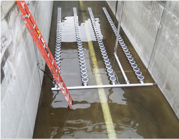
OXIDATION DITCH AT KINGSTON TREATMENT PLANT
