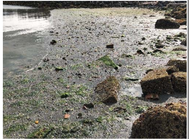
Photograph 4. Looking towards the east at the shoreline area at the base of the riprap revetment.
